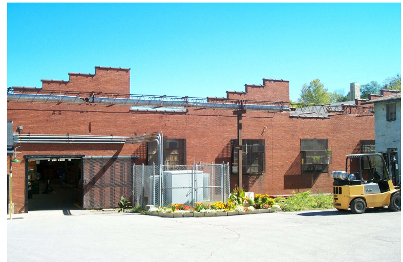
Existing view of South elevation, I-Hall is in the foreground to the right
